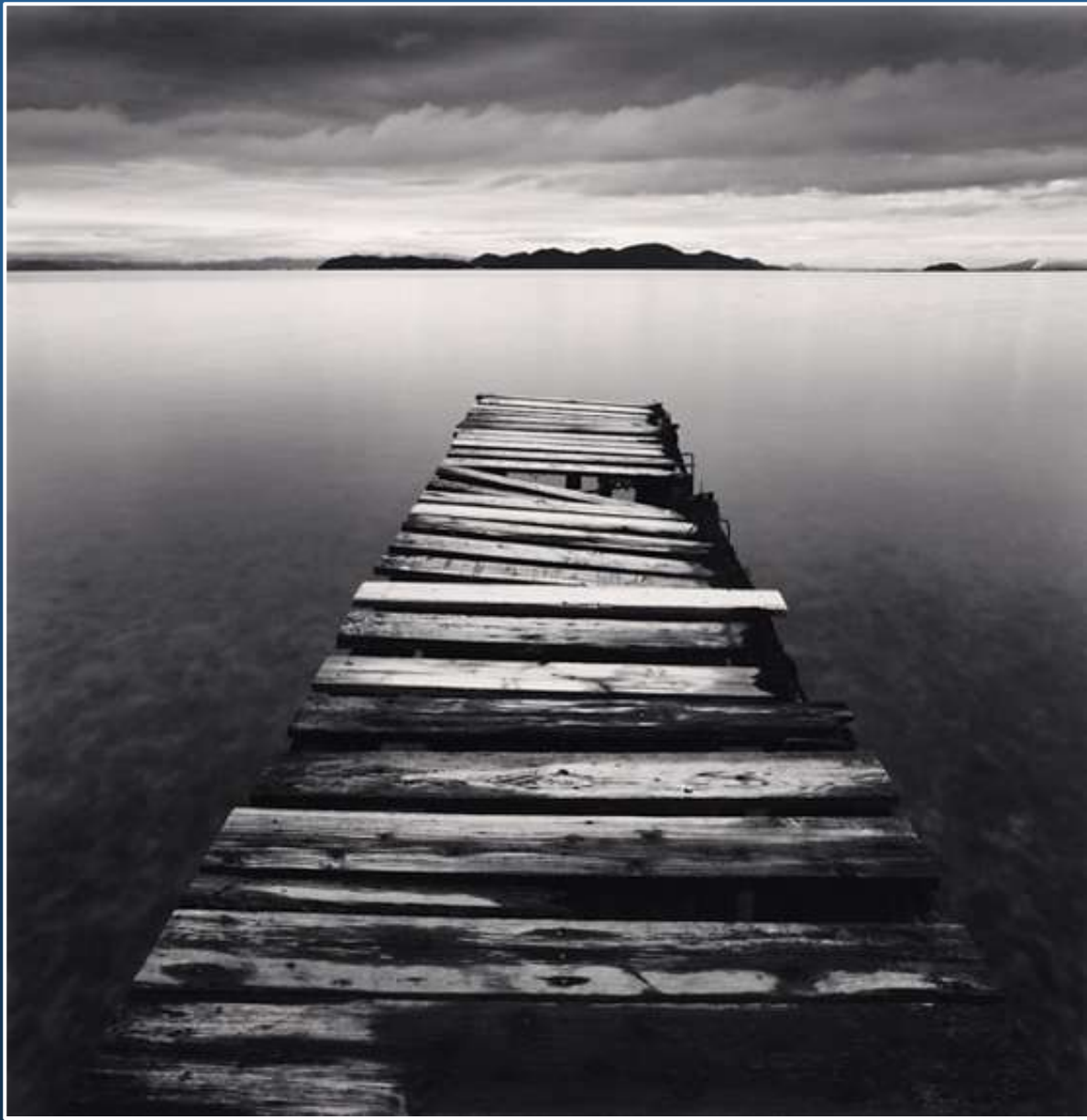
Crumbling Boardwalk, Shiga, Honshu, Japan 2003
